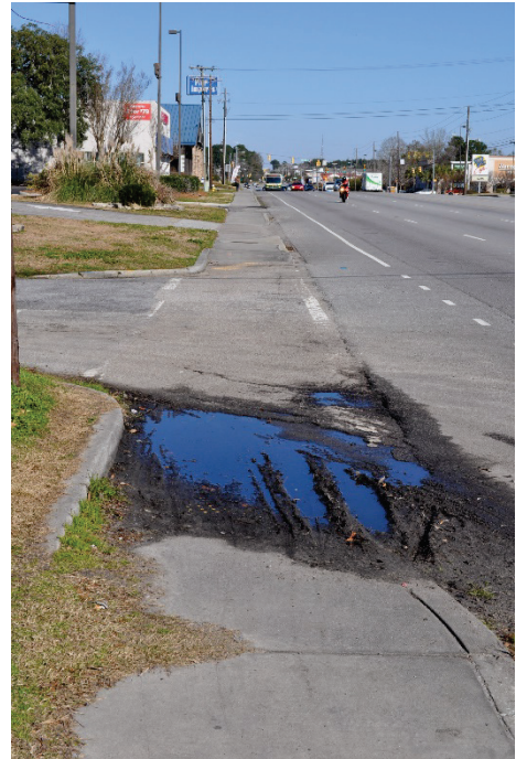
Sidewalk conditions along Rivers Avenue just north of Ashley Phosphate Road
