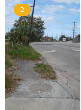
North of Morrison Dr, there is no sidewalk on the west side of Meeting St, and sidewalks on the east side have significant maintenance issues.
