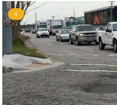
The intersection of Otranto Rd and Rivers Ave is not currently ADA accessible due to slope issues, queuing areas that are too small, and a lack of high-visibility crosswalk markings. In addition, only a small stretch of disconnected sidewalk connect east from Rivers Ave. Addressing these issues would increase the accessibility of the neighborhoods connecting to Otranto Rd.
